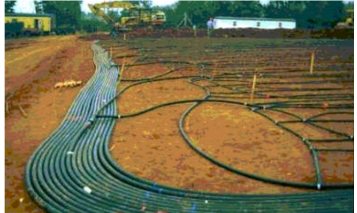
A view of a ground source heat pump used for heating and cooling a home. Photo courtesy of NRCAN
